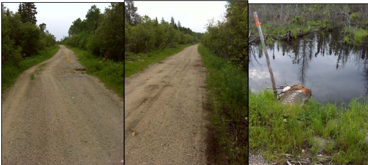
Figure 1. Various areas requiring repair along the Newmarket Concession Road.
